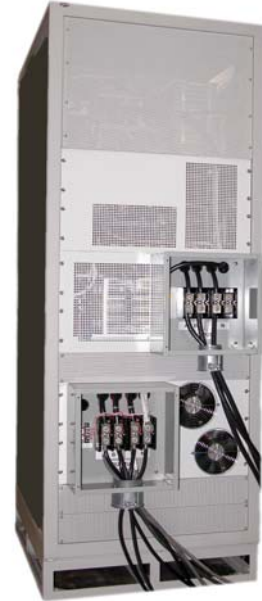
Shown with junction box cover removed
